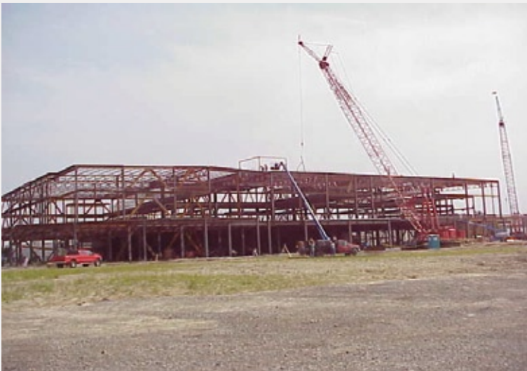
Erecting the structural steel for Westfield Shopping Town at Toledo's Franklin Park
