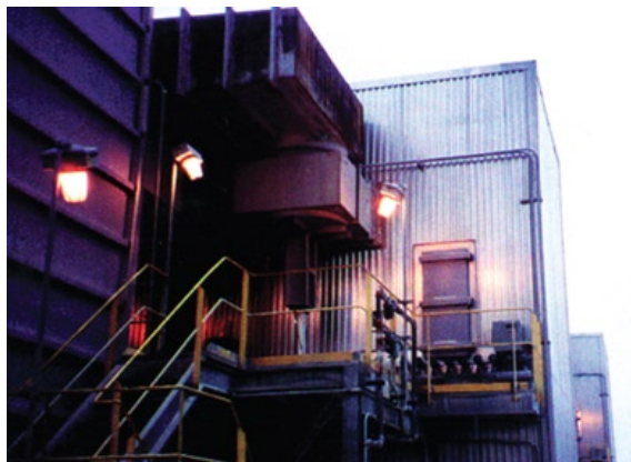
HTH installed the insulation and lagging on this mixing tower at a chemical processing plant
